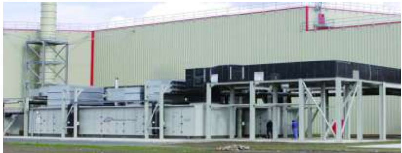
Stringers packaged AirCHP Energy Centre
